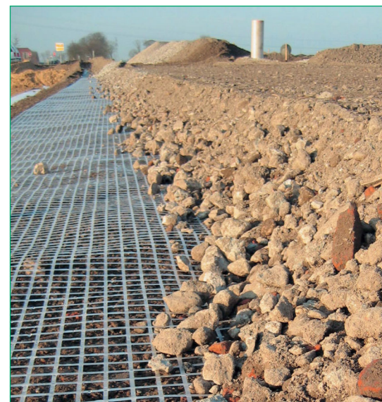
Fig. 19 Crushed base course material over geogrid for base stabilisation in access roads
